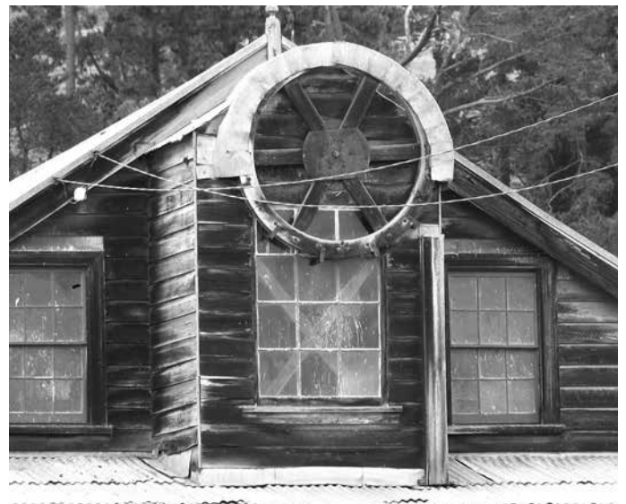
A closer view showing a distinguishing feature – the wheel for the lifting tower which hoisted wool bales to the upper level for storage in the loft.
